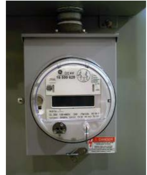
Source: NREL PIX #07805
