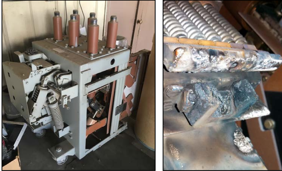
Figure 3: Old main switch with melted contacts
