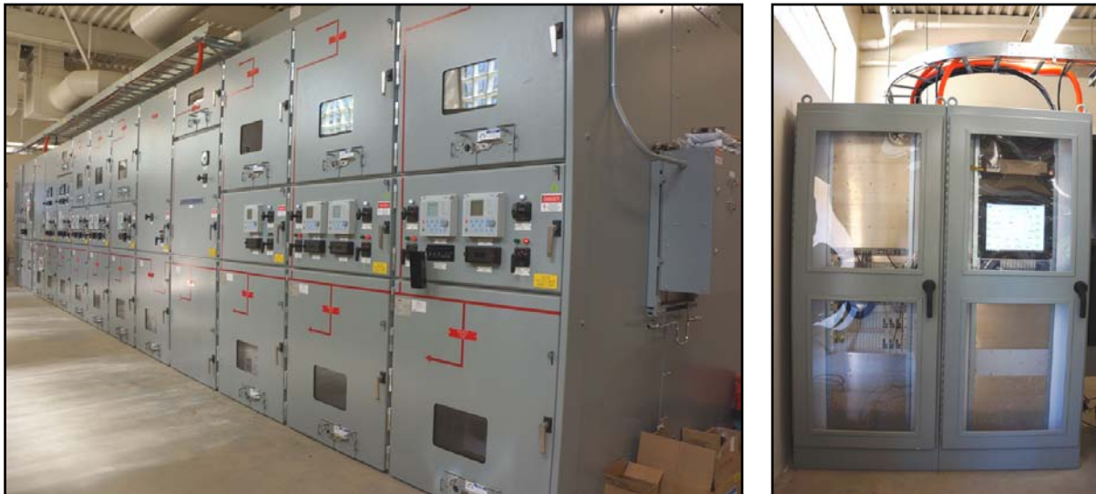
Figure 9: 12kV metal-clad switchgear lineup and control cabinet racks in switchgear control building
