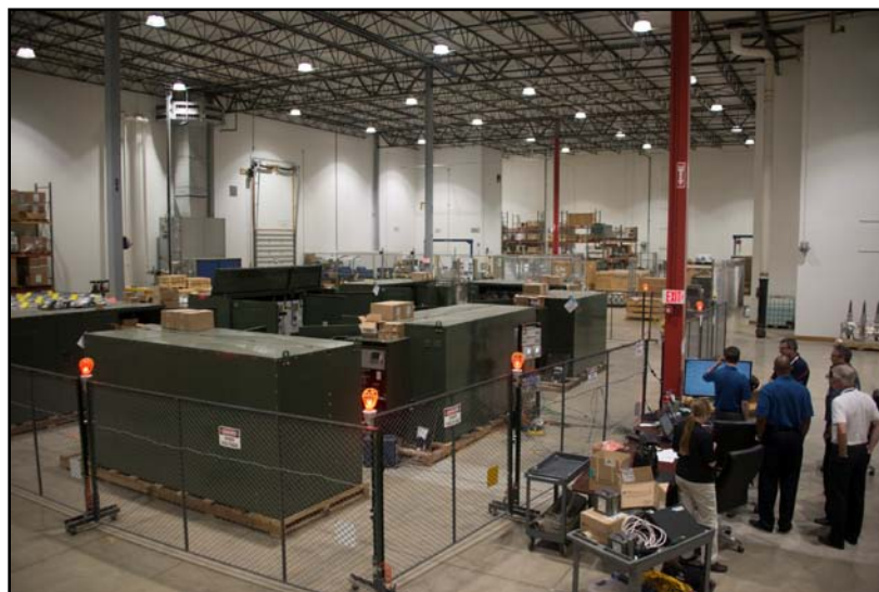
Figure 12: Factory Acceptance Test for complete automation solution
