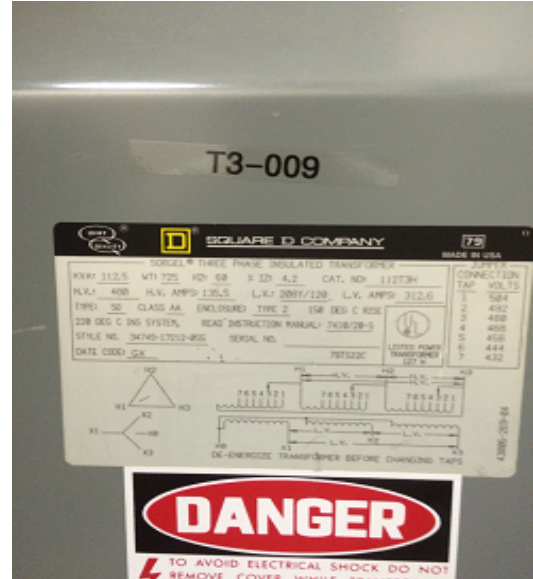
Figure 4: Square D _Nameplate
