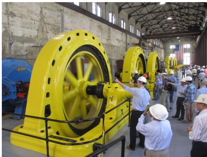
Figure 1: The Mechanicville hydroelectric power plant - generator hall
