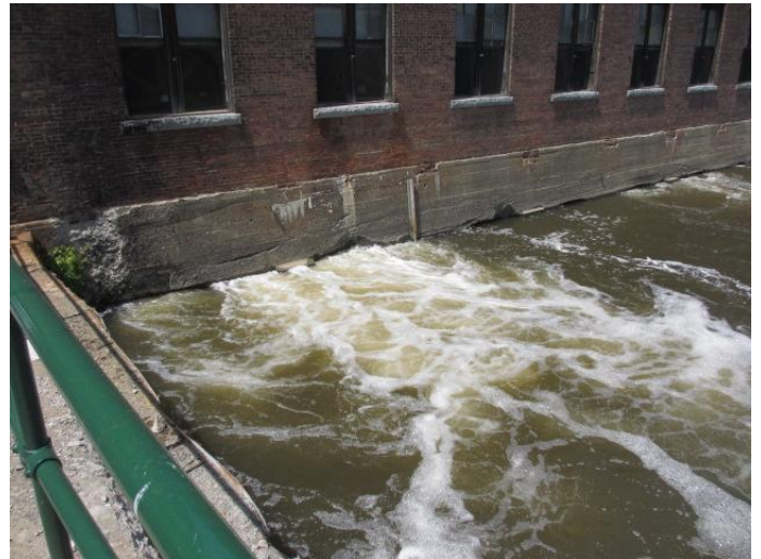
Figure 3: Turbulence in the water discharged from the power house
