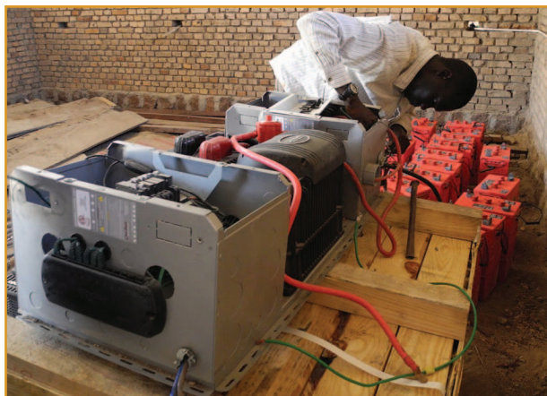
figure 2. Installation of the CCS in Thiou, South Sudan (photo courtesy of Mou Riiny).
