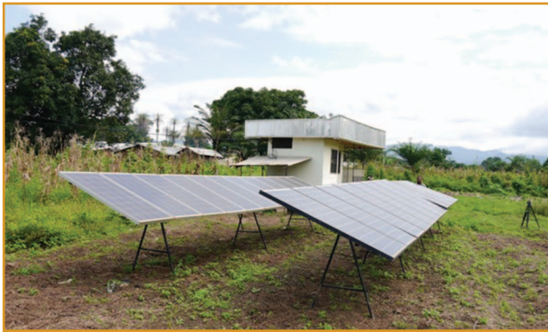
figure 1. PV panels at the Sabongari CCS in Cameroon (photo courtesy of Michael Wilson).
