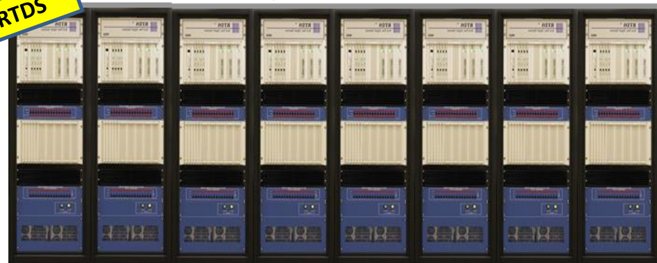
Rack 1 Rack 2 Rack 3 Rack 4 Rack 5 Rack 6 Rack 7 Rack 8
