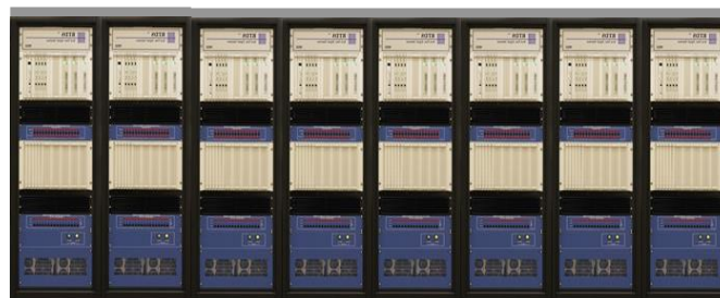
RTDS with 35 Racks
