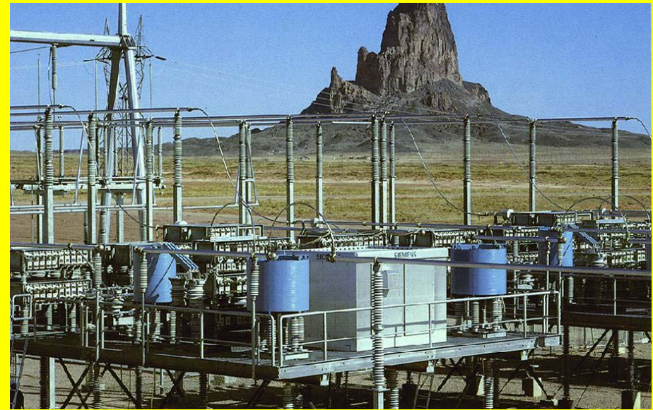
Thyristor Controlled Series Capacitor
