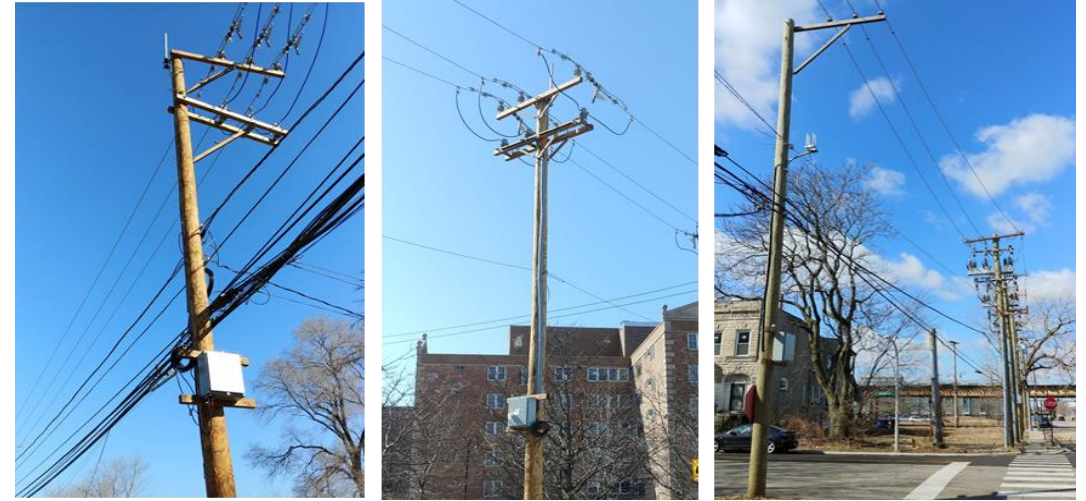
SIMPLE 1, SIMPLE 3 and the POI cabinet
