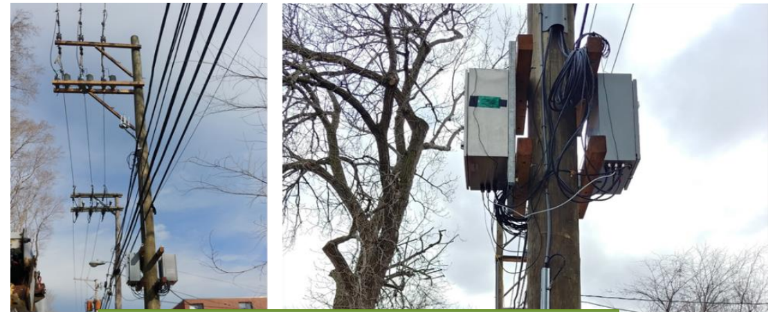
SIMPLE 2 and MVCAL Cabinet
