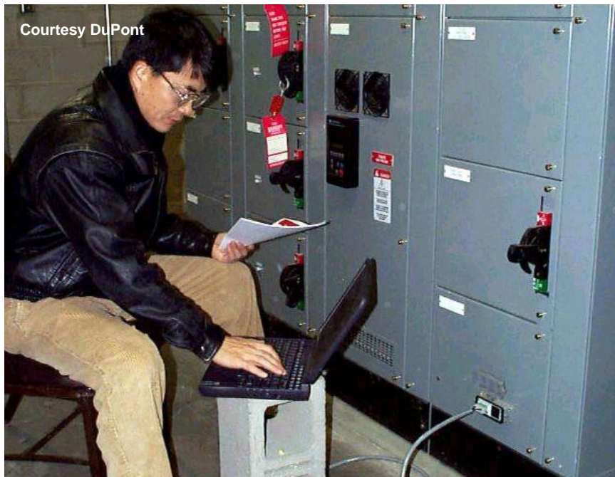
Smart MCC troubleshooting
