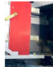
5. Circuit Breaker Approaching Hook
