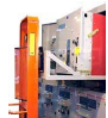
6. Roll Circuit Breaker in Cell
