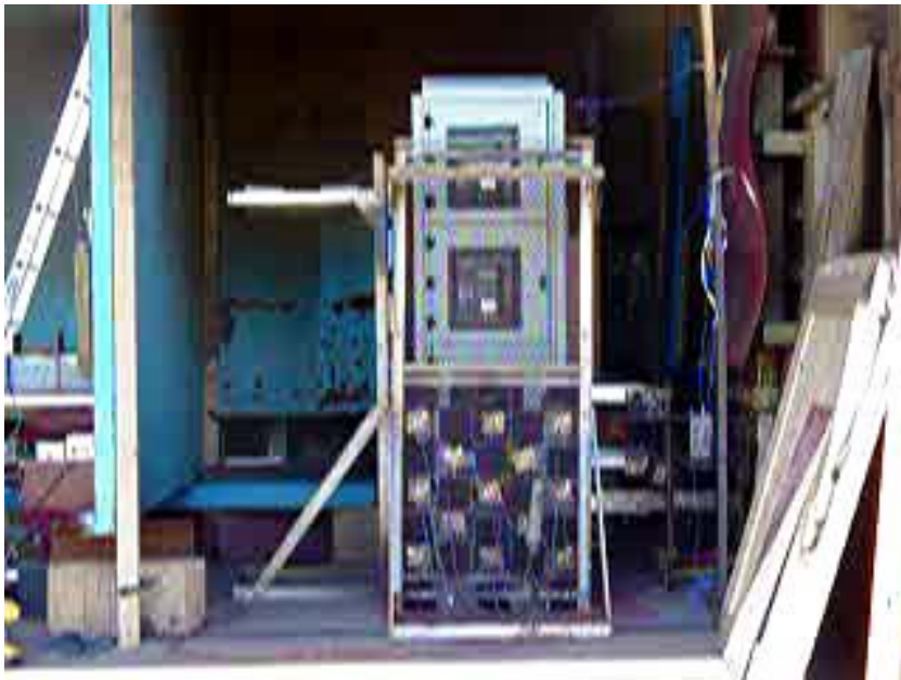
Uninsulated Main Bus 85kA 635V 530msec 63psi 1.5 to 3 cal/cm 2
