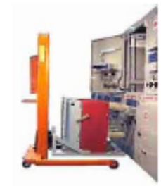
4. Lift Truck & Switchgear Position
