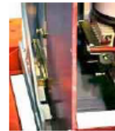
3. Circuit Breaker & Tray Latched in Place
