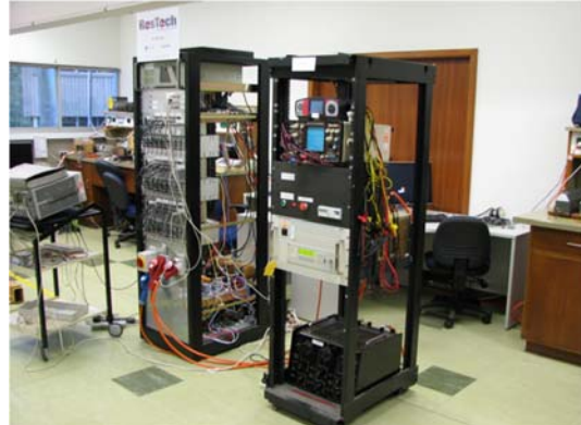
Figure 1. Prototype statcom for power quality improvement in mining.
