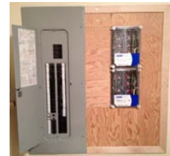
Collecting data from multiple breakers
