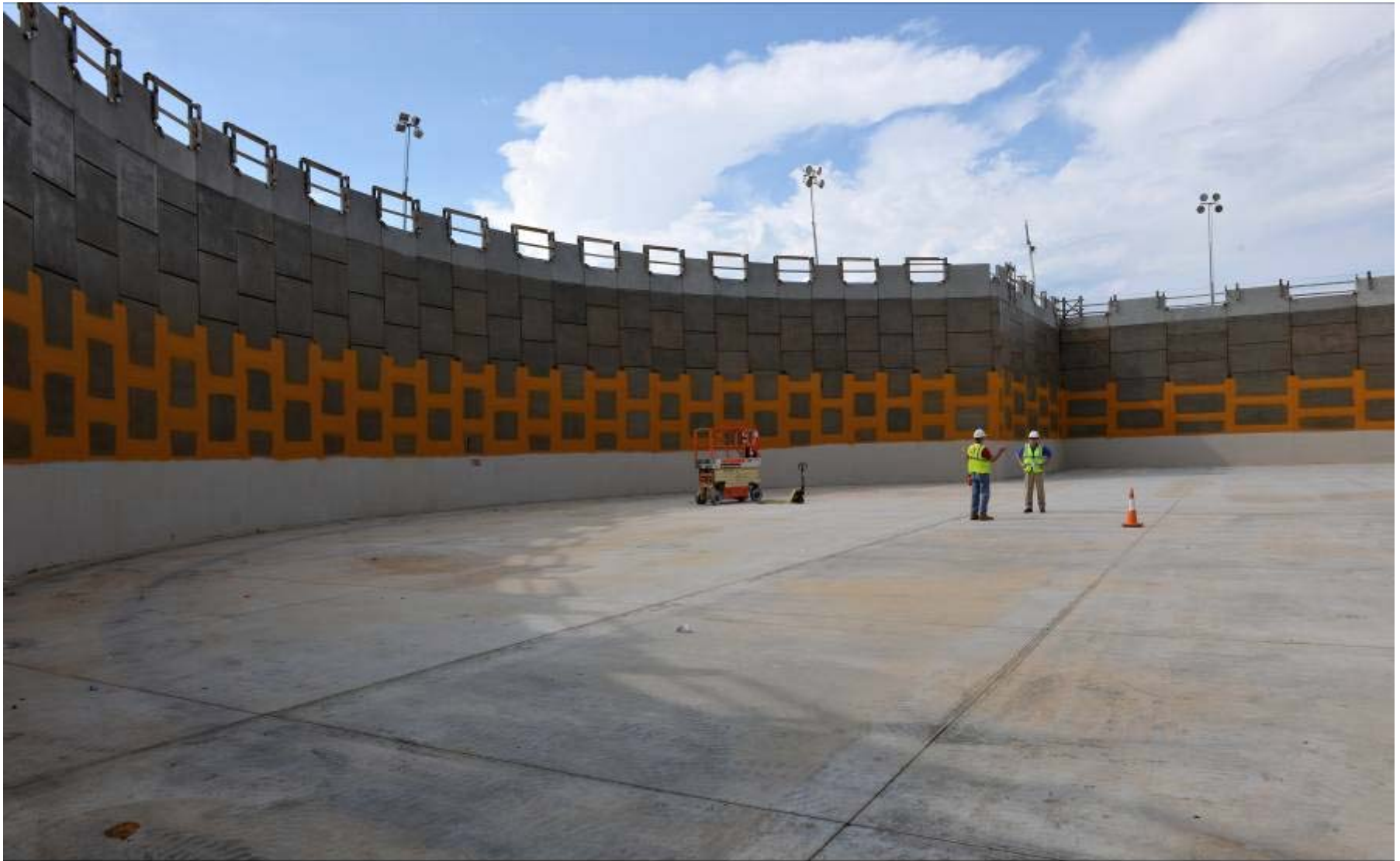
Vogtle Unit 3 "nuclear island," with water proofing work in progress; location where containment vessel and associated nuclear components will be placed.
