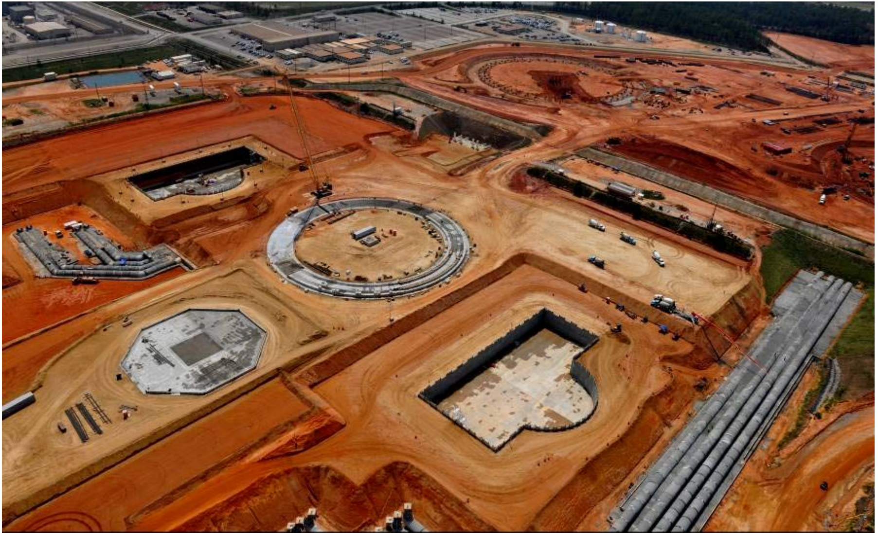
Aerial photograph of Vogtle 3 and 4 construction site. Unit 3 is located at left and top of photo and Unit 4 to the right and bottom. Heavy lift derrick crane foundation in center. August 11, 2011
