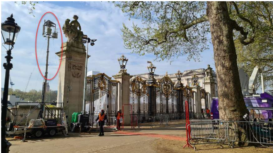
Figure 6.4: Popup n77 private 5G network mast (circled in red) serving the area just in front of Buckingham Palace.
