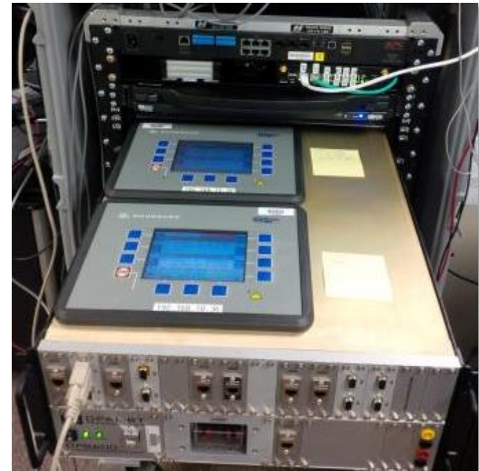
Two integrated Woodward easYgen 3000 genset controllers
